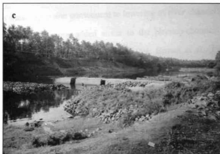
Plate 3: Field photographs from Periyar and Chalakudy basins (a) Cluster of industries in the Periyar basins; (b) An arm of Idukki reservoir near Cheruthoni (Periyar river basin); (c) Check dam constructed in the Chalakudy river near Chalakudy town.
